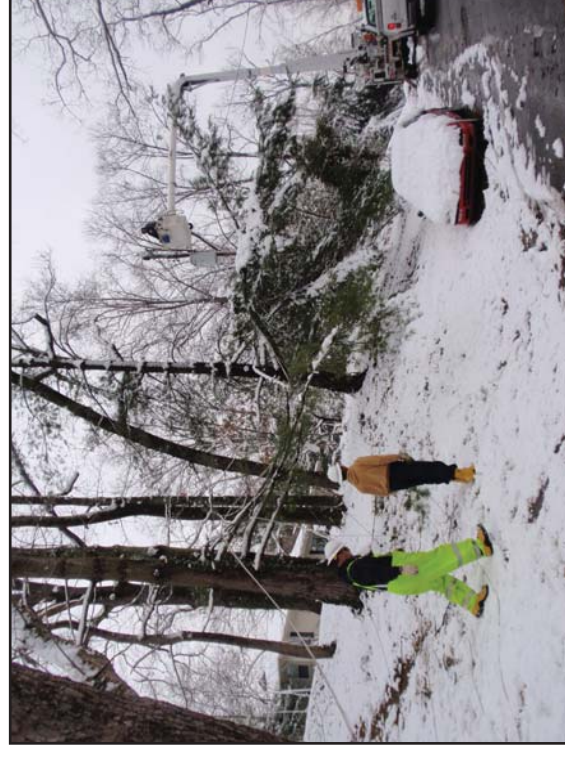
Crews had to be extra careful as many power lines had fallen and were lying on the ground. YOUR SAFETY is very important to us. NEVER touch a power line that has fallen to the ground. Immediately call 282-JCPB to report.
